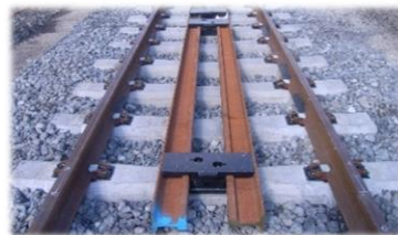
Derailment prevention guards
